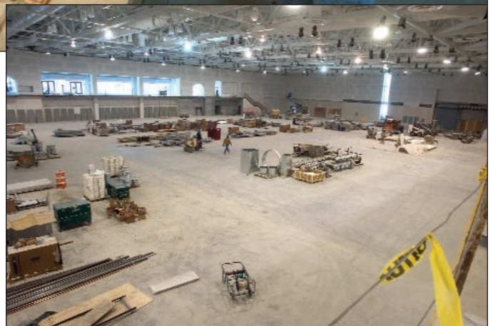
Top: Jonathan Hoffman '01 (civil engineering technology), a project engineer for The Pike Co., observes work on the competition pool in the new Gordon Field House and Activities Center. Above: The facility’s multi-purpose area will accommodate 8,000 people.
