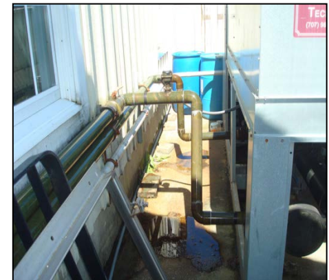
Heat Loss on Chiller Pipes
