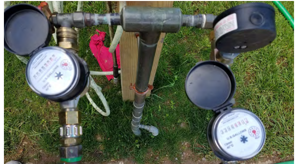
Image 3: Flow meters attached to wash station hose
