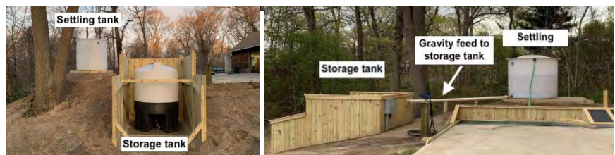
Image 17 (LEFT): Side view of Version 2 showing settling tank above storage tank; excavating was required to place the storage tank at a lower elevation. Image 18 (RIGHT): Full view showing gravity feed pipe connecting two tanks.
