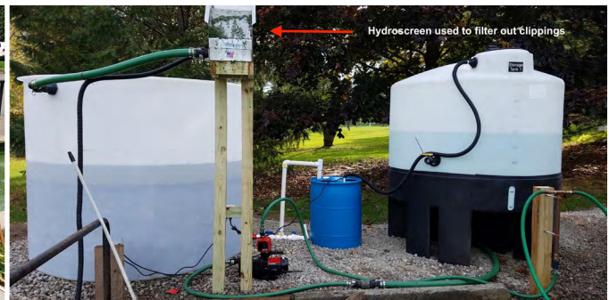
Image 8: External hydroscreen to filter out excess clippings
