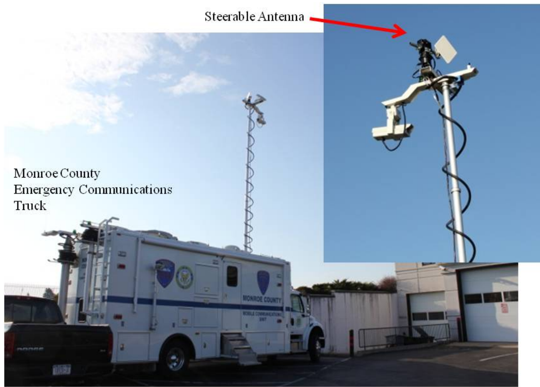
Figure 3.10-28: An example of the portable ground station, as installed on the Monroe County Emergency Operations Communications Vehicle.
