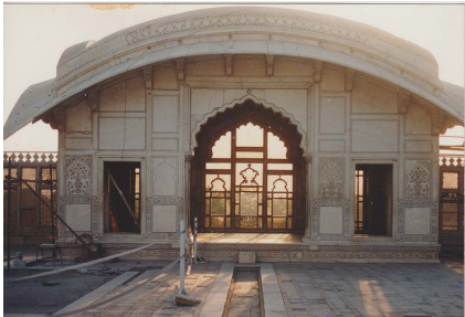
Fig. 1. An image of the Naulakha or Queen's Pavilion, a monument inside the Lahore Fort. It's dilapidated condition speaks to the challenges faced during physical restoration
