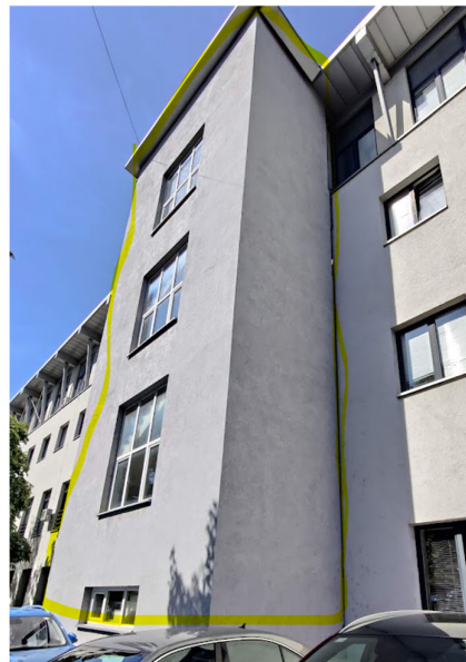
Old staircase object for removal
