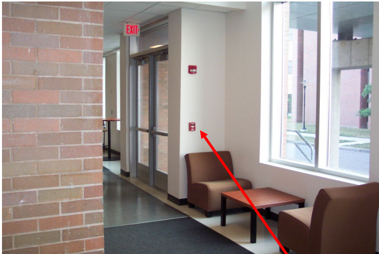
Fire alarm pull-box Outside NW Exit
