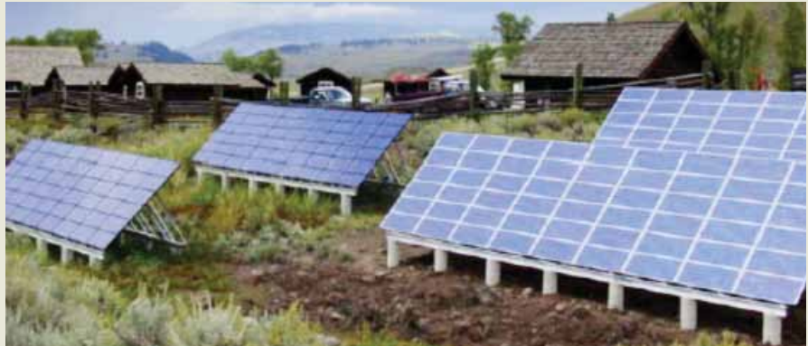
Ft. Stanwix National Monument: Renewable energy system installed through the University-National Park Energy Partnership Program.
