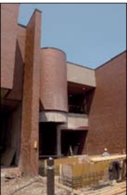
Renovations now in progress will be completed in time for fall classes.
